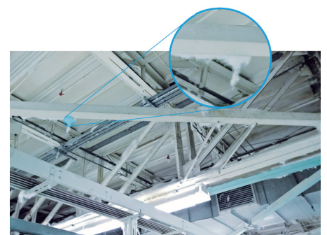
Dust Deposits in Ceiling
